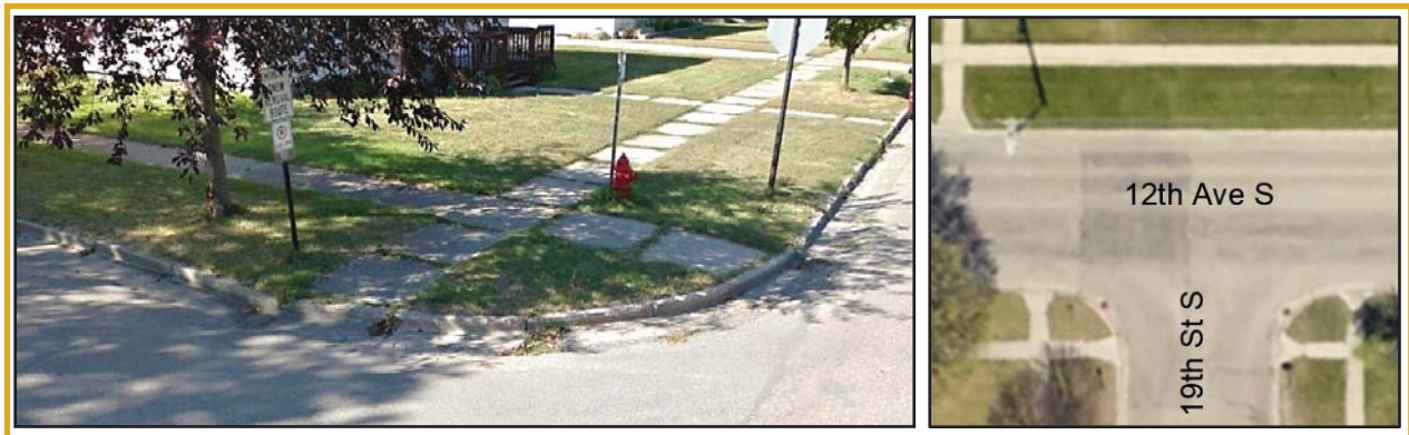
Many Sidewalk Curb Ramps Do Not Meet Current ADA Guidelines or Do Not Align
