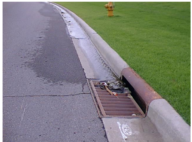
Please help keep storm drains clean. Soil, trash and other pollutants flow untreated, directly to our rivers, lakes and streams.
